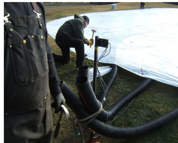
Figure 6. System ready for blower & meter.
